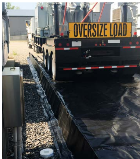
Mobile transformers driven into HardyBerm portable containment system.
